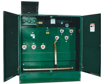
3PH Padmount Transformers
