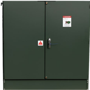
3PH Padmount Transformers
