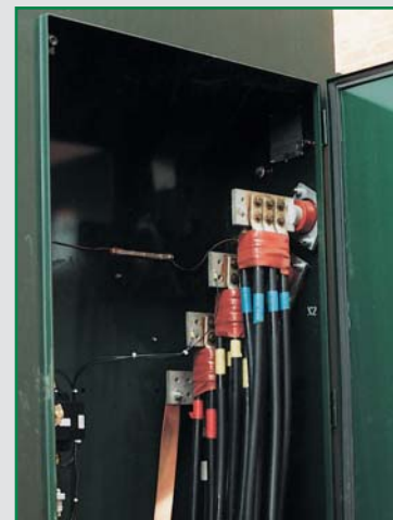
Low voltage compartment
