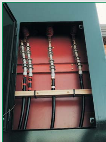
High voltage entrance
